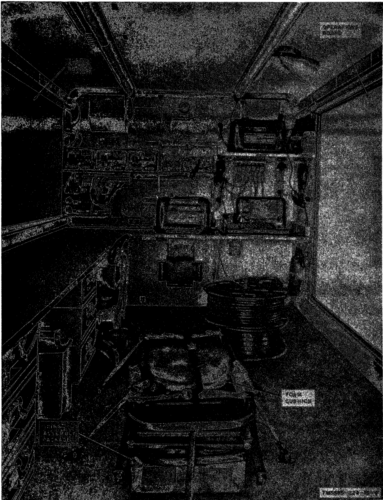
Figure 7. Operations Central AN/MS-32, interior front view.
